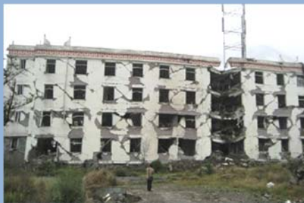
Collapsed dormitory for students (Sichuan)
