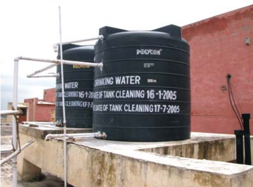
Syntex Water tank at roof without anchorage
