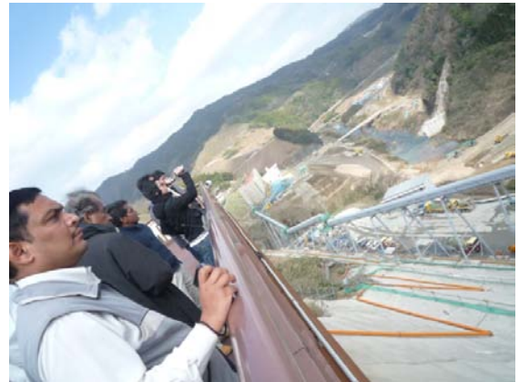
Photo 4-25 Observation at the Obara Dam construction site [Hii River and Kando River General Development and Construction Office, MLIT]
