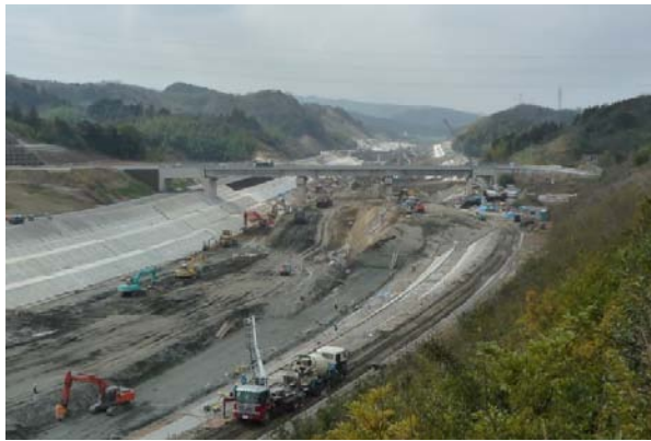
Photo 4-24 Observation of the Hii River diversion channel construction site [Hii River and Kando River General Development and Construction Office, MLIT]
