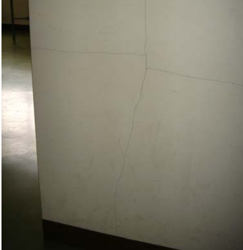
Surface cracks after the earthquake
