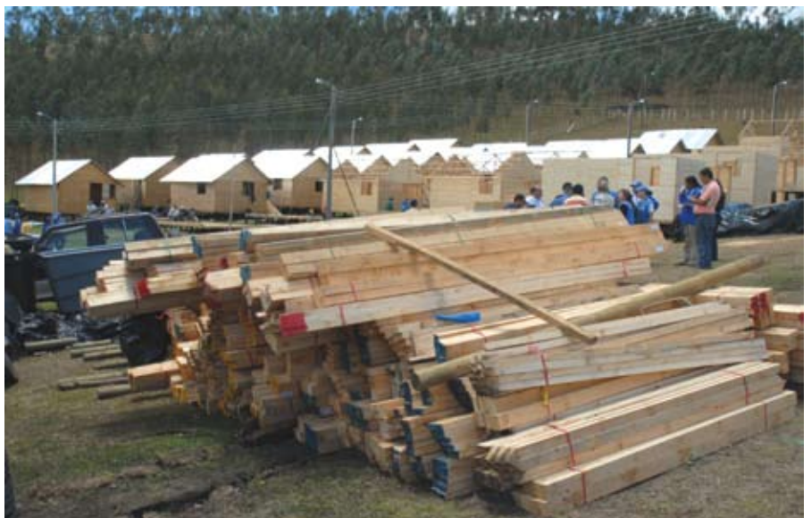
Development of a refuge area in case the Galeras volcano would erupt, Colombia
