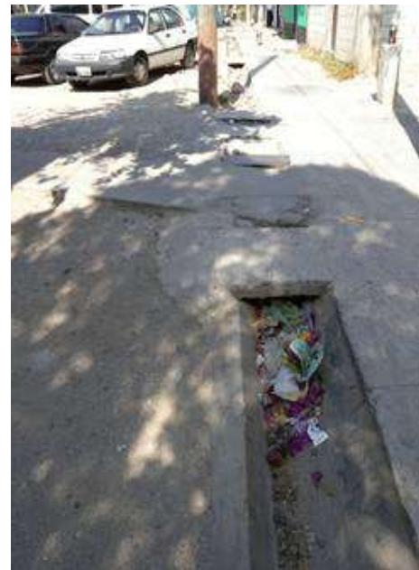
Figure 14. Trash accumulation in drainage ditches.
