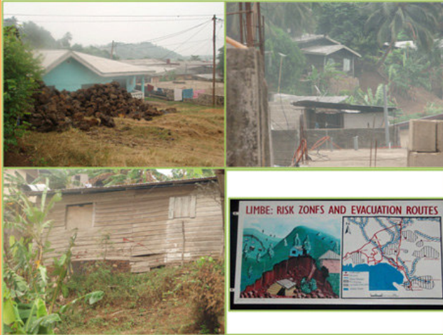
Sample of houses built on landslide body, and an information risk billboard
