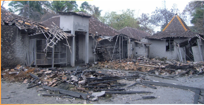
Structural damage to buildings in Bronggang village, Argomulyo. Two timber frame buildings have suffered fires and collapses. The intact nature of tiles on the roofs, along with other evidences, suggests that this surge was associated with relatively low dynamic pressures.
