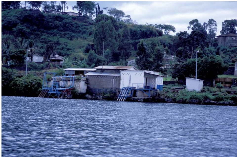
Fig.13. Lake Kivu water pumping station : water intake only metres from lava flow
