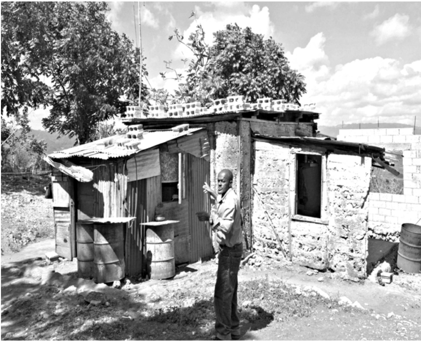
Dennis Thompson surveys his storm-damaged house in Jamaica in the wake of Hurricane Ivan in 2004
