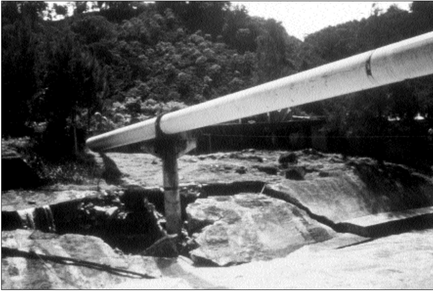
Flood damage to the bridge supporting the main water pipe of the Orosi system in Costa Rica in October 1999. Some 500 tons of concrete were displaced.
