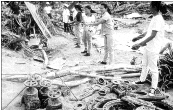
Damage to a water company's storage facility in Tegucigalpa, Honduras, following Hurricane Mitch.
