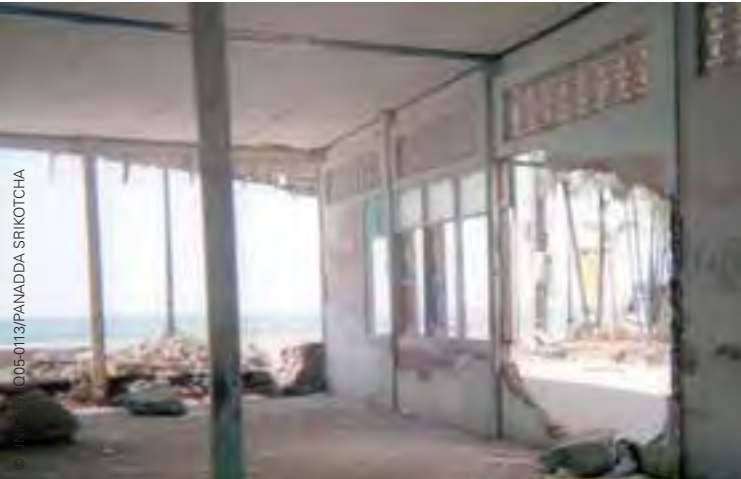
A house that was heavily damaged faces the sea in the Katoo District in the province of Phuket, Thailand. "This is what is left of my house. I feel sorry for my parents who have to work hard to rebuild it," says the photographer, Panadda Srikotcha.
