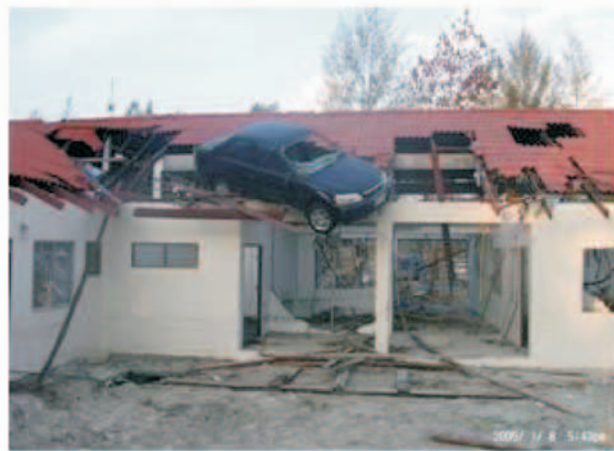
Figure 8. Tsunami damage photos of commercial/government structures in Phang Nga: (a) Completely destroyed Bamboo Orchid Resort; (b) Heavily damaged Similana resort; (c) Heavily damaged Phang Nga government building.
