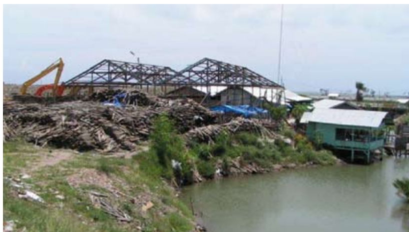
Figure 12: Wood recycling at Gampong Jawa dumpsite as part of the Tsunami Recovery Waste Management Programme.
