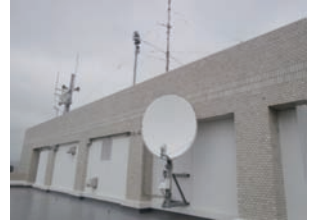
Figure 5. Antenna and studio installed at the Natori City hall
