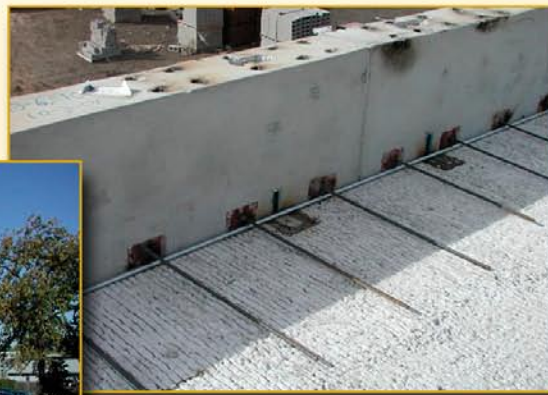
Connection between precast concrete wall panels and roof. Special inspections are necessary during construction for all shelters. For shelters built with wall panels, special attention is required to ensure that the connections between the wall panels and the roof and foundation are properly made.
