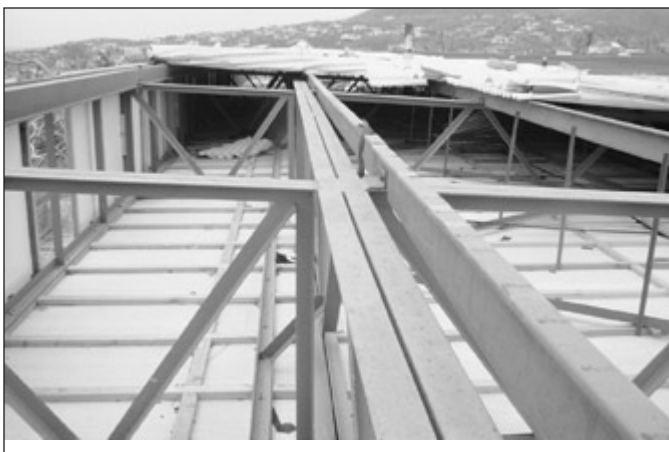
Although the structure was undamaged, the widespread loss of roof sheets in a hurricane meant that the hospital was effectively unuseable. (Photo Tony Gibbs)
