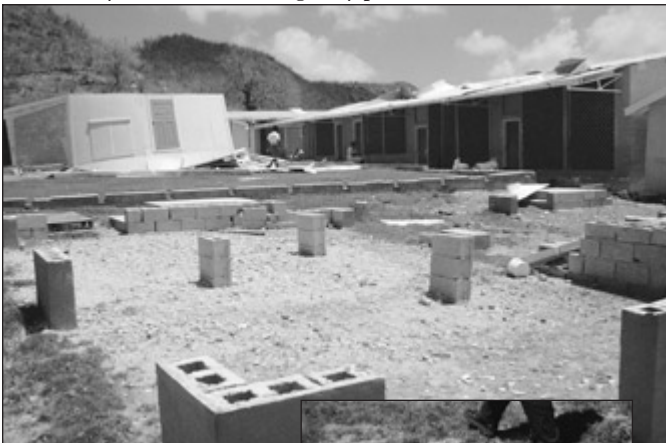
The absence of anchorage led to the removal and overturning of the entire building of this clinic in a hurricane. (Photo Tony Gibbs)
