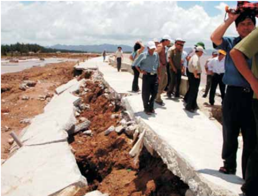
Damage caused by the Damrey Typhoon in July 2005 to Hai Hau in Nam Dinh Province.
