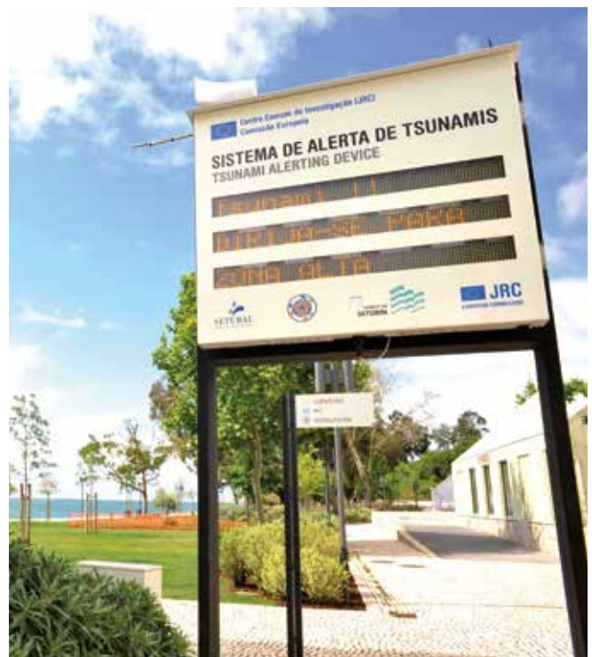
Tsunami Alerting Device (TAD) in Setubal (Portugal). Testing is performed in collaboration with the local Civil Protection authorities.
