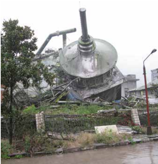
A collapsed drier at a fertiliser plant after the 12 May 2008 Wenchuan earthquake.
