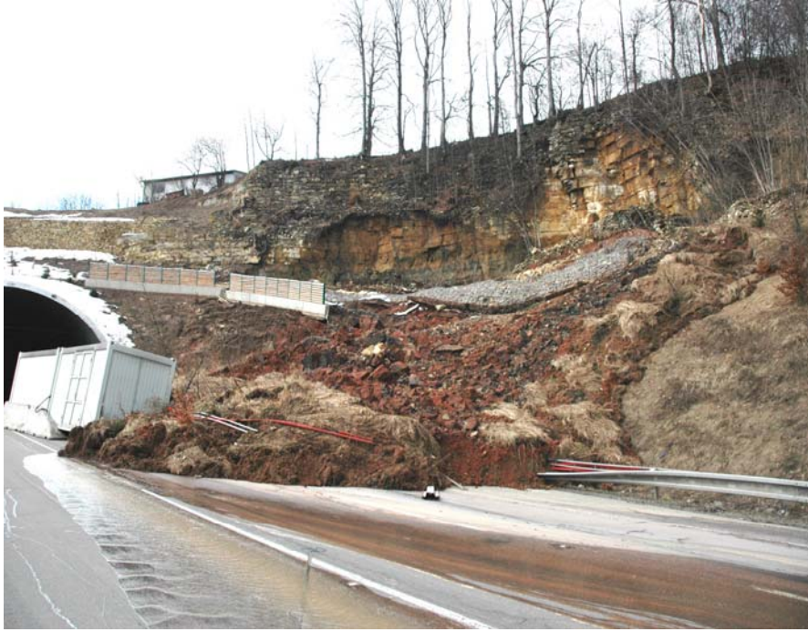
Figure 2: The Hrebec landslide, Czech Republic, March 2006- situation during the first day of the origination (Source: Oldrich Krejci, Czech Geological Survey)
