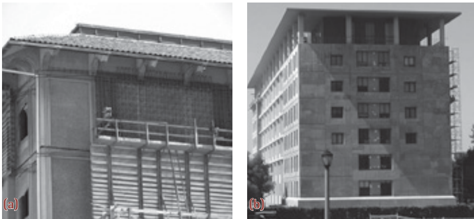
Figure 14.6. (a) Retrofit work, Berkeley University Campus (b) Barrows Hall, Berkeley University Campus
