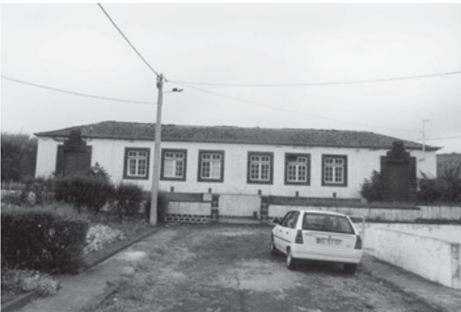
Figure 8.6. Dislocated roof tiles at Castelo Branco (Carreira) school
