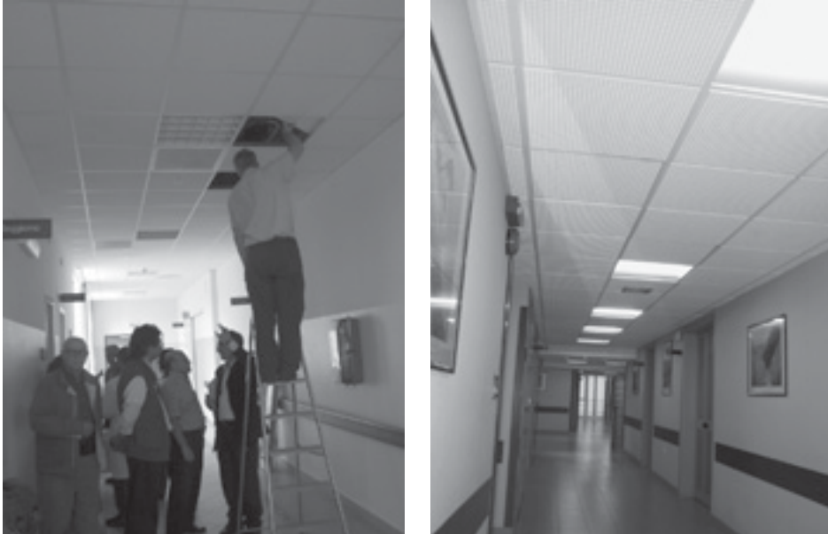
Figure 12.2. Seismic characteristics and recommendations for a suspended grid ceiling in Italian hospitals
