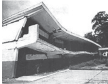
(b) Structural collapse in longitudinal direction of Valentín Valiente School (Bonilla et al., 2000)
