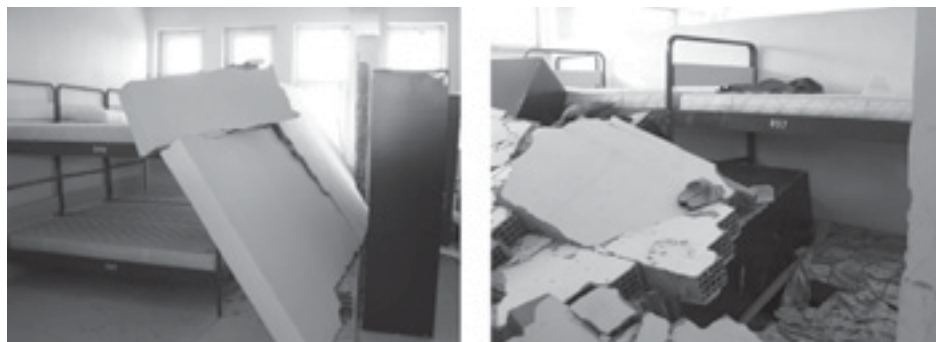
Figure A4.12. Collapse of free-standing masonry walls onto beds in dormitory buildings
