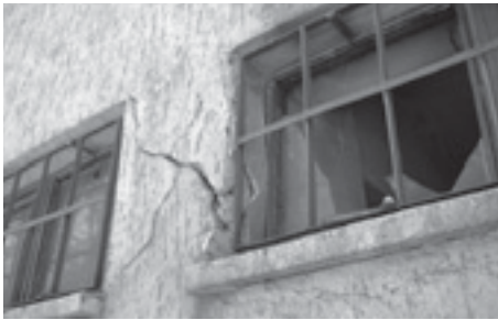
Figure A4.5. Shear failure of captive columns created by the small windows of the furnace room in building C-14-03
