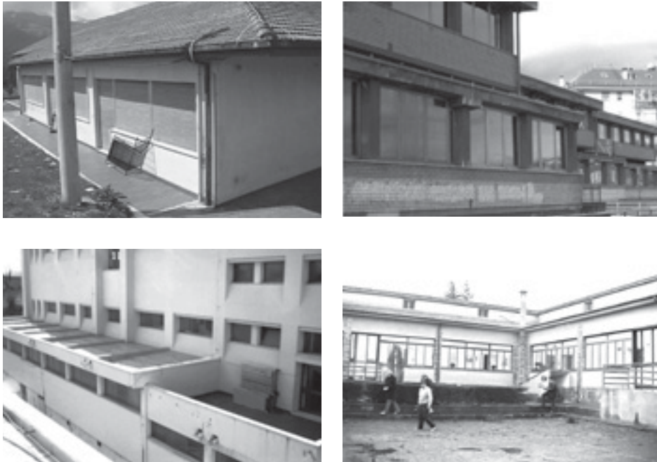
Figure 3.4. Wide windows, large inter-storey drift, irregular shapes of single- and multi-storey schools
