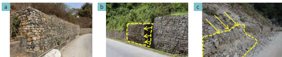
Figure 2: (a) refers to retaining walls judged to be undamaged in the damage survey, (b) to those that were partially deformed or bulged out, and (c) to those that had collapsed.
