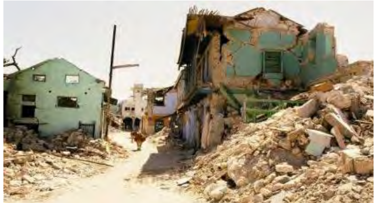
Figure 1. Masonry Collapse in Gujarat, India (Photo by K. Meguro, 2002)
