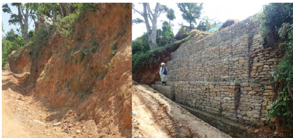
Figure 5. State of Test Construction of Gabion Retaining Wall before and after Construction
