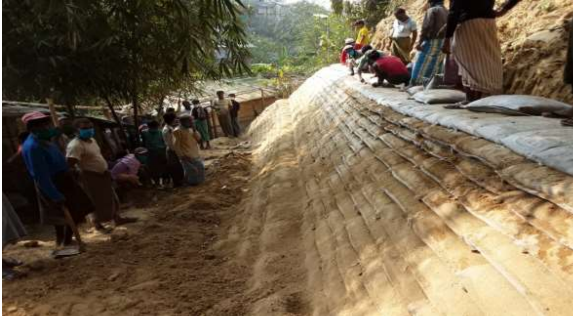
Photo: Disaster Risks Reduction Construction Work for combating landslides, Rohingya Camp, Cox's Bazar, ICCO, 2020
