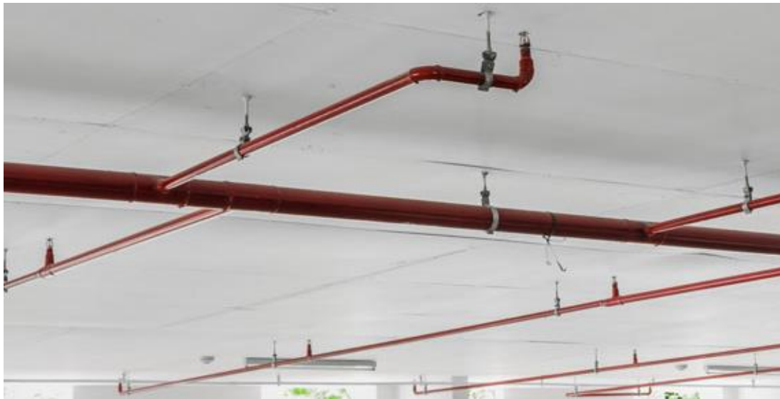
Automatic Sprinkler System
