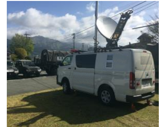
To introduce approx. 100 additional vehicle-mounted mobile phone bases to enable major base stations to continue providing service in an emergency
