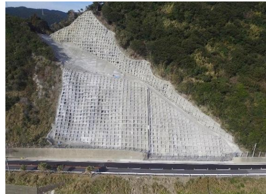
To reinforce road slopes and embankments and expand road widths at approx. 2,000 locations prone to landslide
