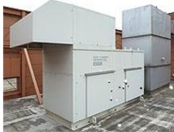
To support 125 disaster-medical and other hospitals in introducing in-house power generation systems
