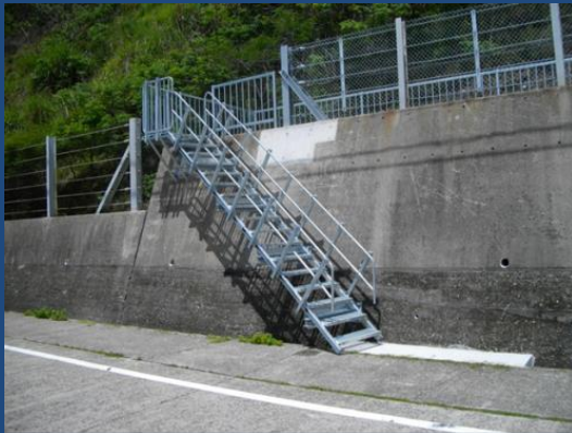
Emergency evacuation stairs (Sumoto Nadaka Shusen (Sumoto City))
