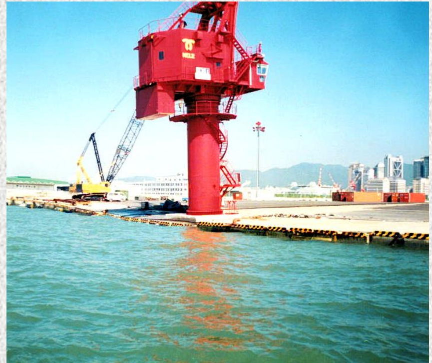
Damaged Quay Wall
