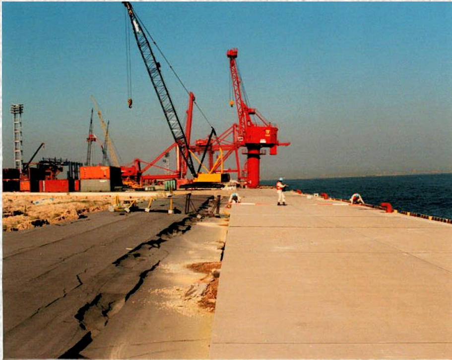
Damaged Container Yard
