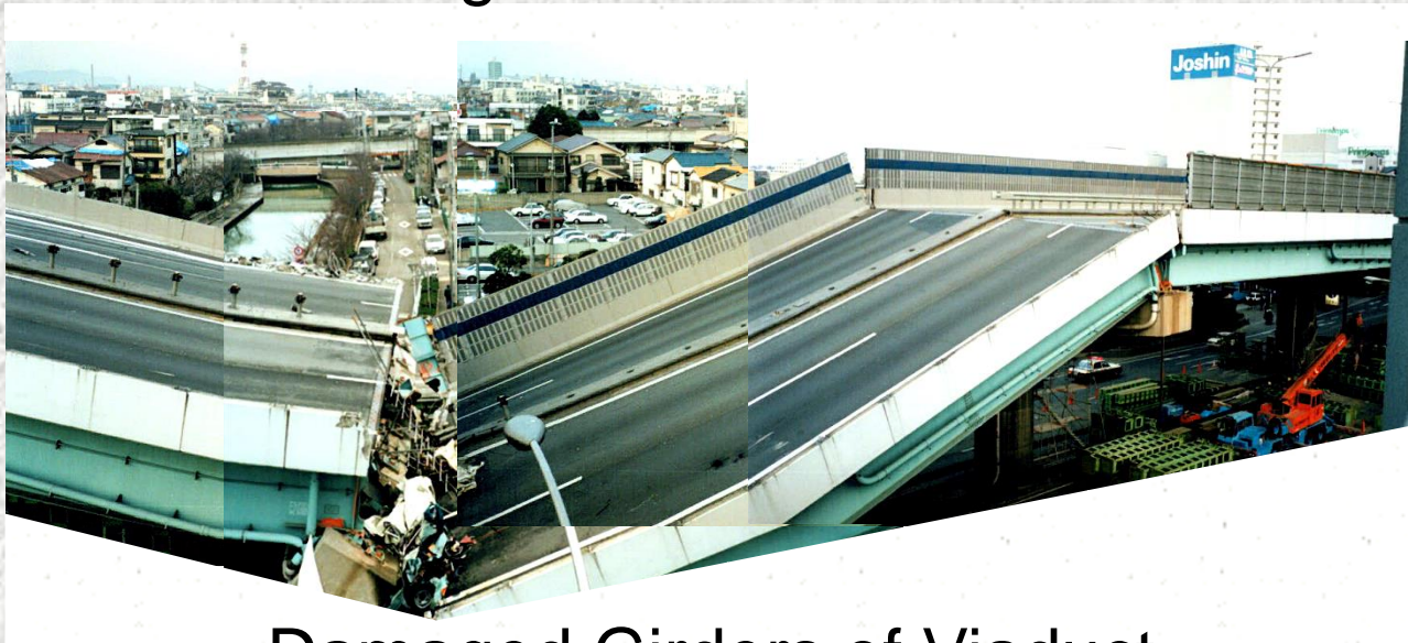
Damaged Girders of Viaduct
