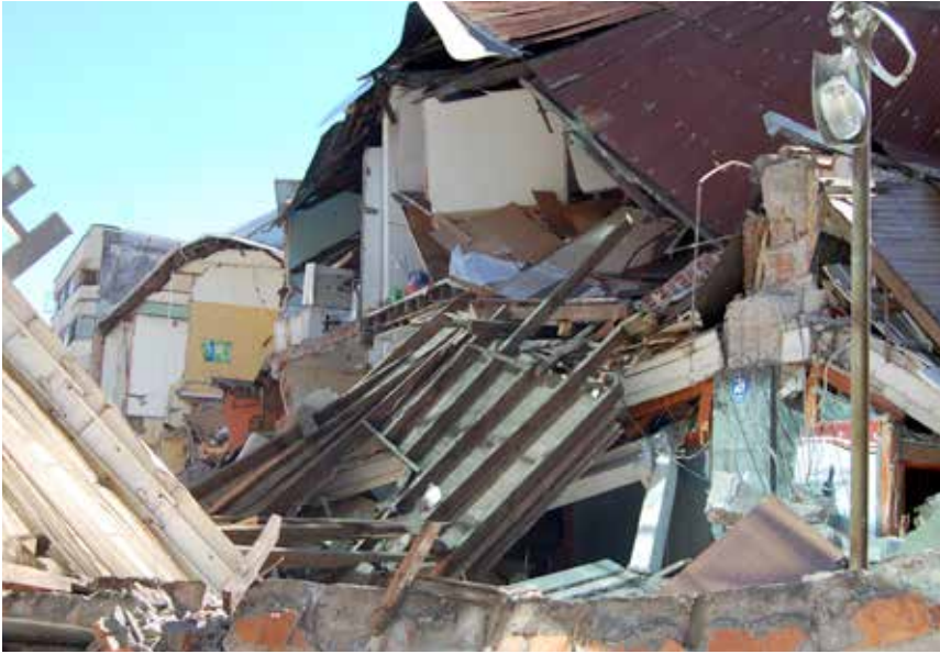
Damage done to houses by the 2010 earthquake with 8.8 magnitude in Concepcion city, Chile. © Shutterstock
