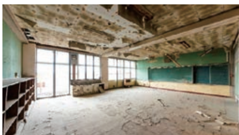
Disaster Memorial Ruin Arahama Elementary School
