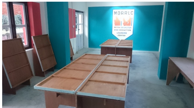
Finally, the top later of exhibit spaces are fitted. The room also contains other display boards.
